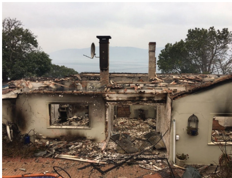
The fires in Knysna and Bitou have caused immeasurable damage and losses to housing
